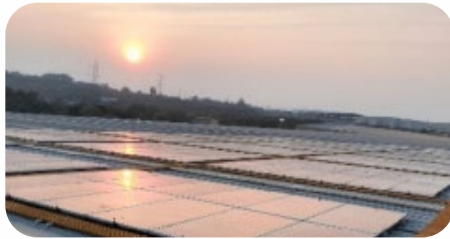
On-site solar roof system
